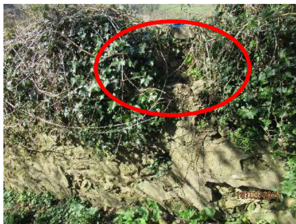
Image showing loss of stone at top of the wall
