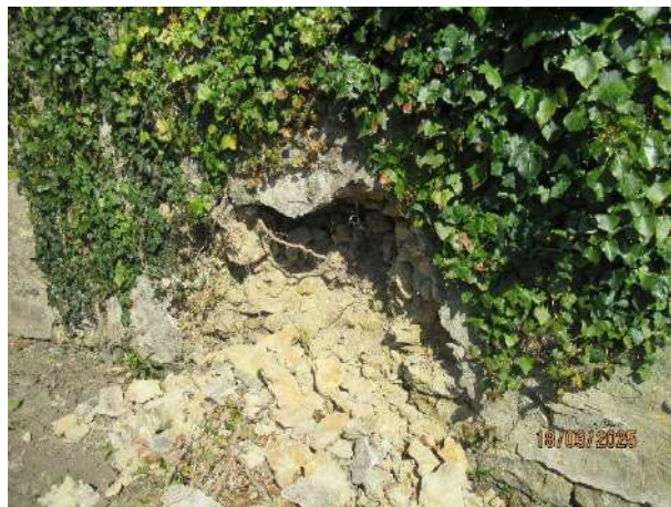
Images showing loss of material at sample areas to the wall
