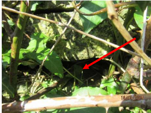
Image showing part of 50mm gap in wall
